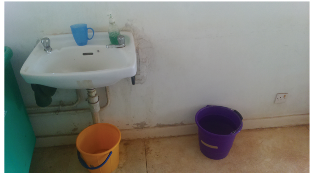
Hand-Washing Facility in the Ward
