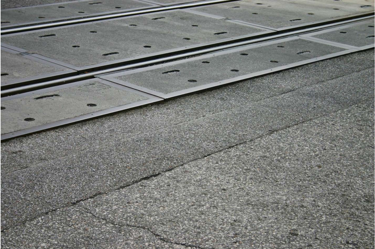
Figure 97. West Approach of Crossing 817405M with Uneven Crossing Surface, Close Up
