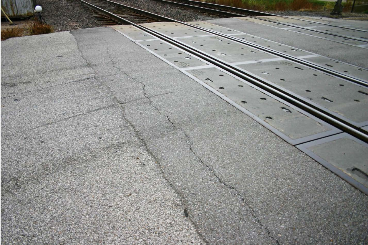
Figure 102. East Approach of Crossing 816134F with Scrape Marks on the Asphalt, Close Up
