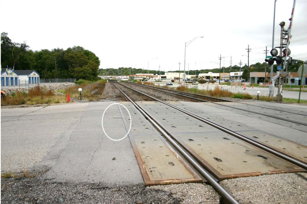
Figure 99. West Approach of Crossing 816134F with Scrape Marks on the Asphalt
