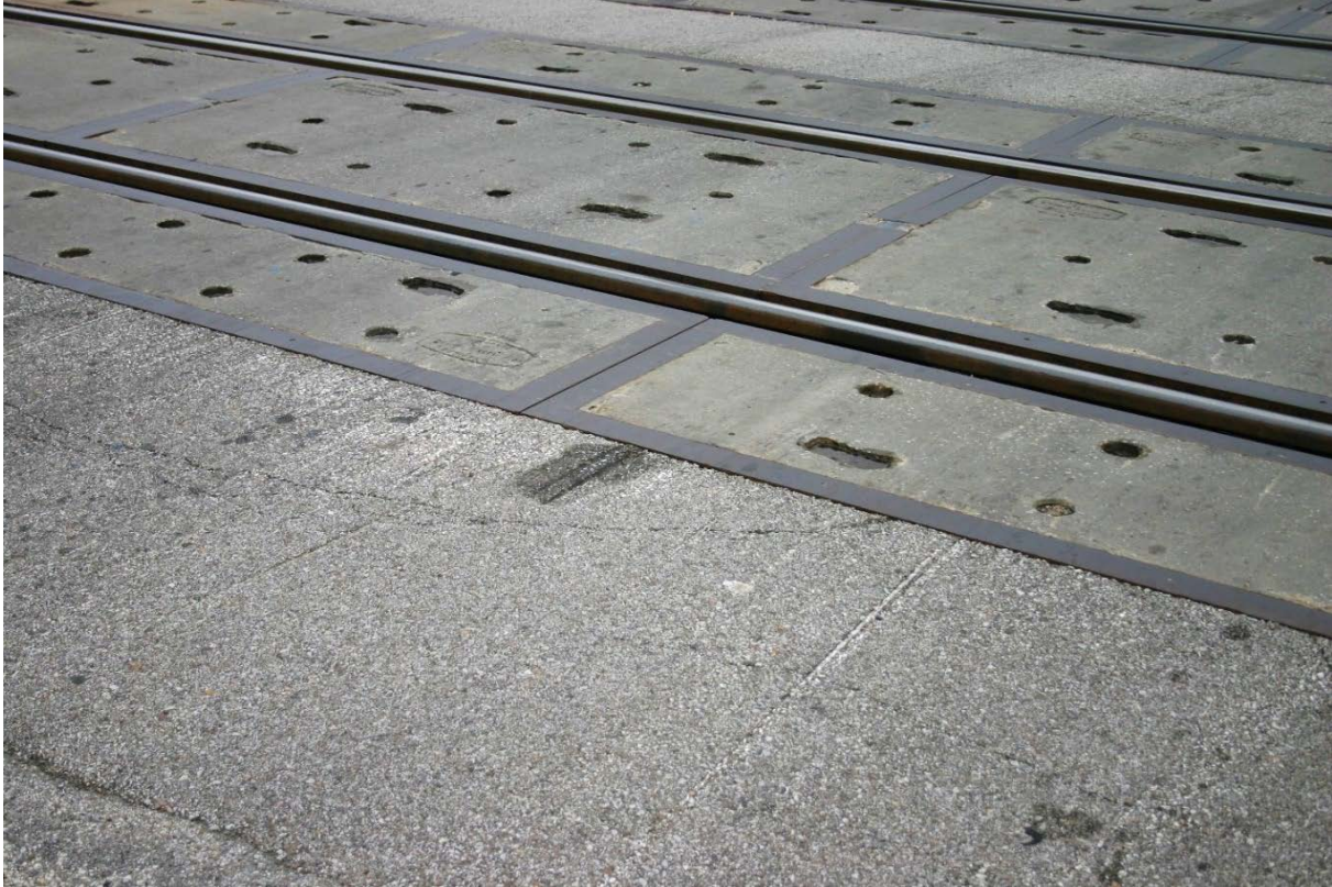
Figure 100. West Approach of Crossing 816134F with Scrape Marks on the Asphalt, Close Up
