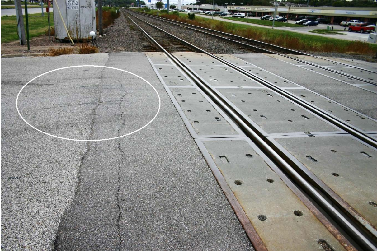
Figure 101. East Approach of Crossing 816134F with Scrape Marks on the Asphalt
