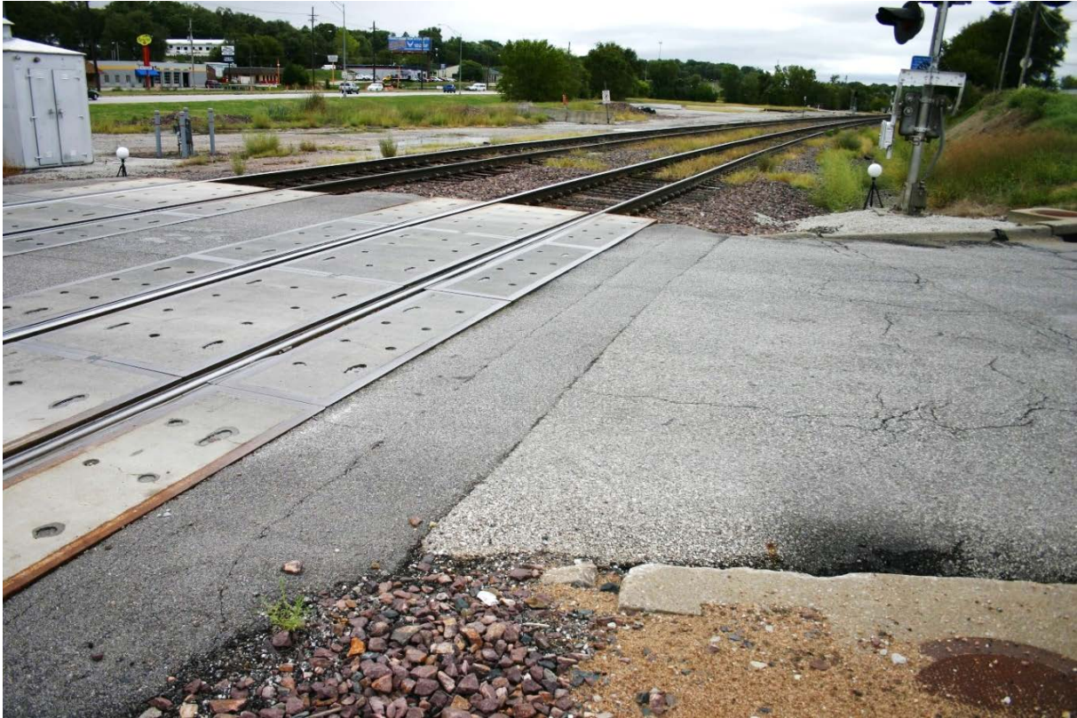
Figure 96. West Approach of Crossing 817405M with Uneven Crossing Surface
