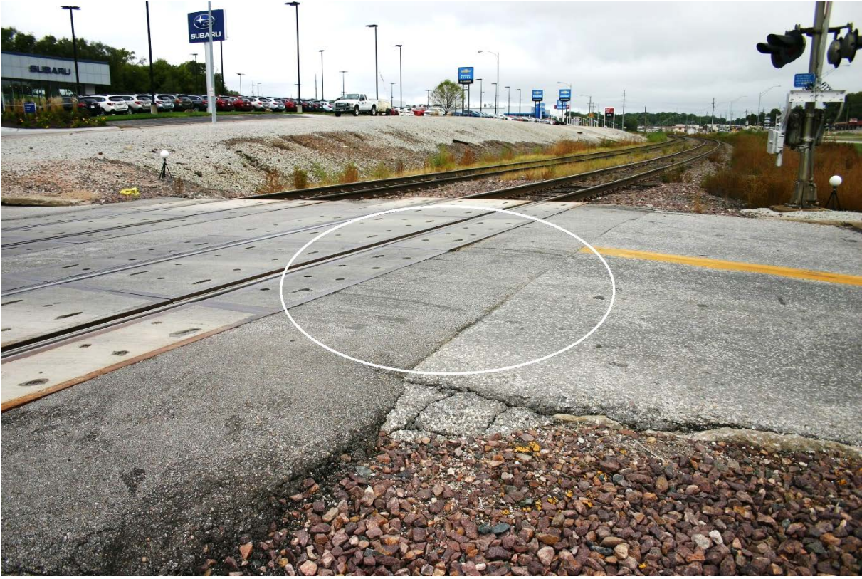
Figure 94. East Approach of Crossing 817405M with Scrape Marks on the Asphalt
