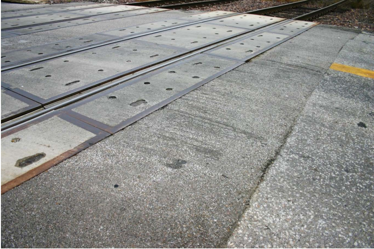
Figure 95. East Approach of Crossing 817405M with Scrape Marks on the Asphalt, Close Up
