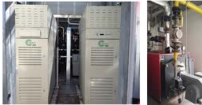
Figure 4. Microturbines (left) and one boiler (right) of the SPM [35].
