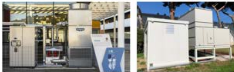
Figure 5. Absorption chillers of the SPM [35].
