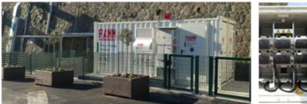
Figure 6. Electrical storage system of the SPM [35].
