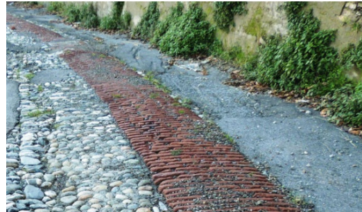
Fig. 4. Cambered profile of the central brick strip and lateral cobble-stone channel (Source: Fratini).
