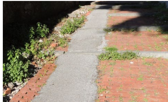
Fig.6 The installation of water systems has damaged the paving (Source: Fratini).
