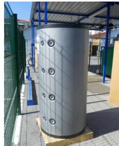
Fig. 5 Thermal Energy Storage
