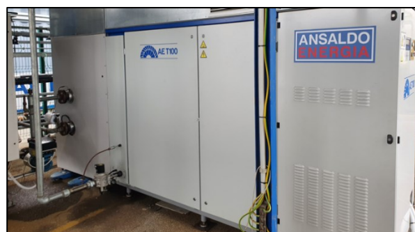
Fig. 4 CHP unit installed at the Campus - external side
