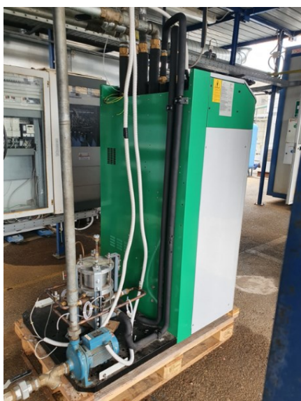
Fig. 3 Innovative HP installed at the Savona Campus
