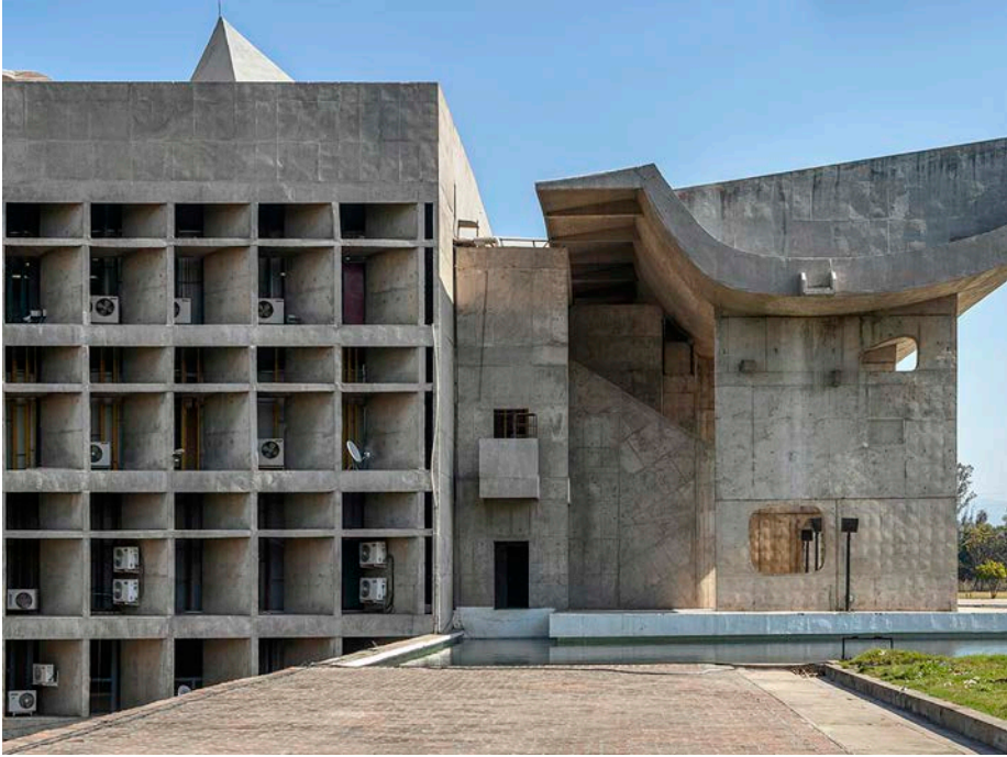
fig. 1. Palace of Assembly in Chandigarh (Le Corbusier, 1951-62), designated as a UNESCO World Heritage Site in 2016. External units of the air conditioning system on the façade. (© Roberto Conte, 2019)
