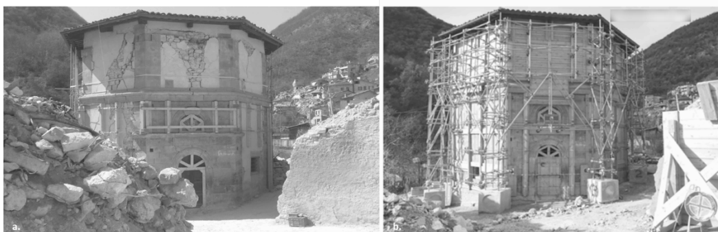
Fig. 5. (a) The church of ‘Madonna del Sole’ after the earthquakes of October 2016; (b) The church in November 2017.
