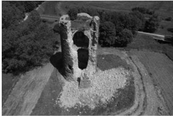
Figure 2. Virgin Tower at Zichem, an abandoned medieval four stage dungeon erected in the 14th century, after its partial collapse in 2006 due to loading by roof breakdown, important soil deposit and long-lasting water infiltration. The structure has since been consolidated in its present form and protected against further infiltration. The present study deals with the standing walls not affected by the collapse.
