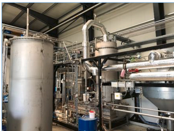
Fig. 9. Hot gas filter and condensation stage of the product gas train of the TCR-500 plant.
