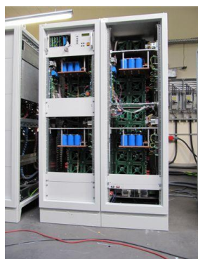
Fig. 4: single power stage of the three phase 240 KVA supply
