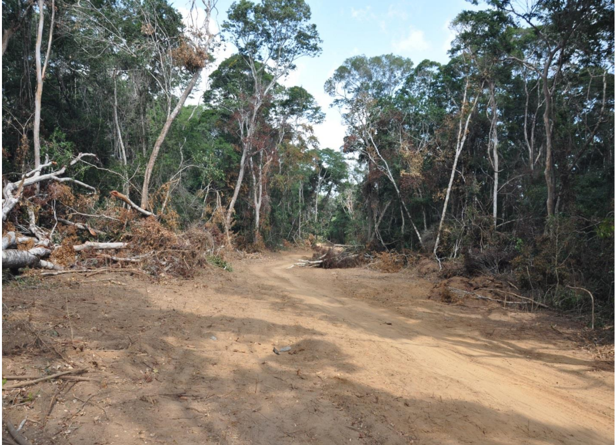
Photo 2: A section of the widened road under construction in Zaraninge forest reserve in SANAPA
