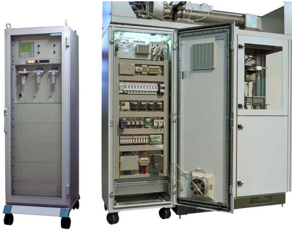
Figure 6. Front and backside (in a cone calorimeter unit) of the gas analysis rack
