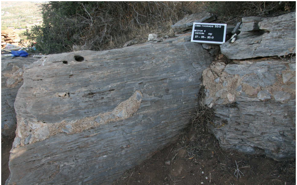
Fig. 15. Cistern no. 1. Fissures in the rock filled with a mixture of stones and lime mortar (2010).
