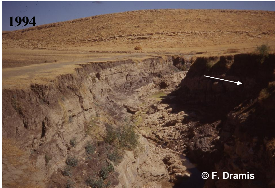
Fig. 4. The gap in the gully bank in 1994 indicates the occurrence of large slab failures (arrow). Note the increase in shrub cover after 1994 on the slope in the background.
