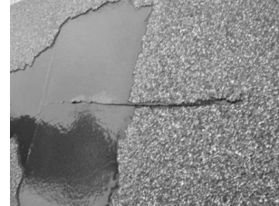
Fig. 3. Longitudinal crack through the deck plate at a stiffener-to-deck plate connection
