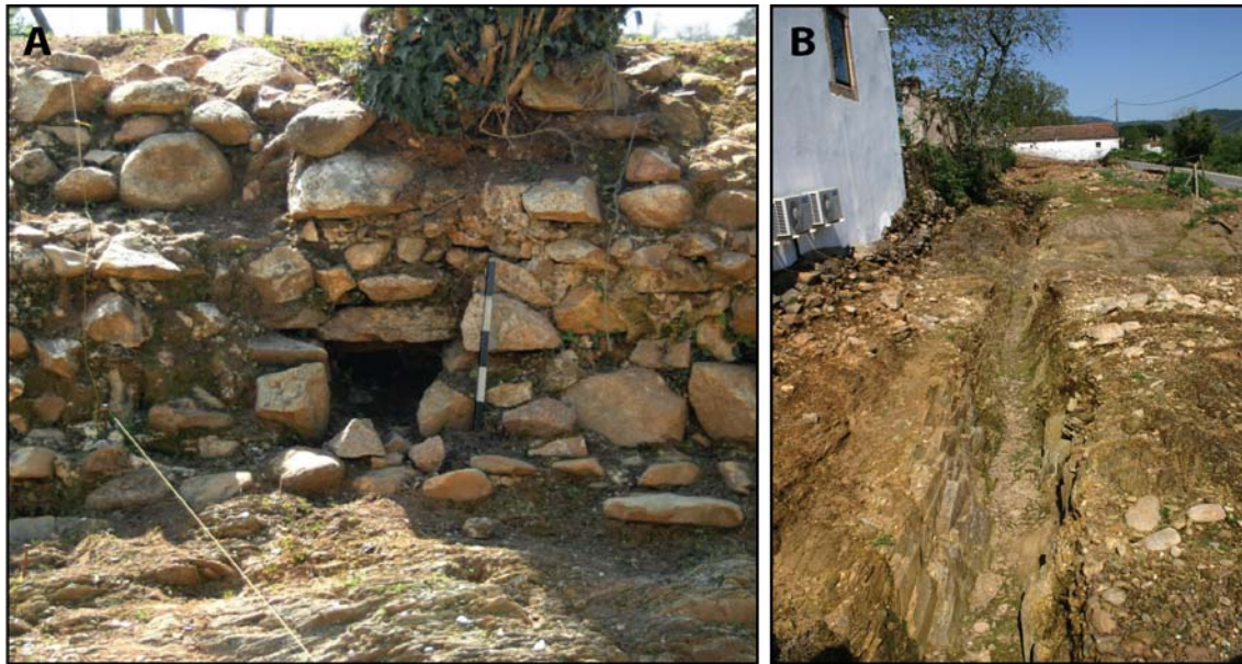
Figure 4.41 (A) Sewer opening in the town wall in the area of insula 38 (scale: 50 cm); (B) V-shaped ditch serving as the main drainage channel for the town. Photo-A by J. Carvalho, photo-B by S. Deprez.
