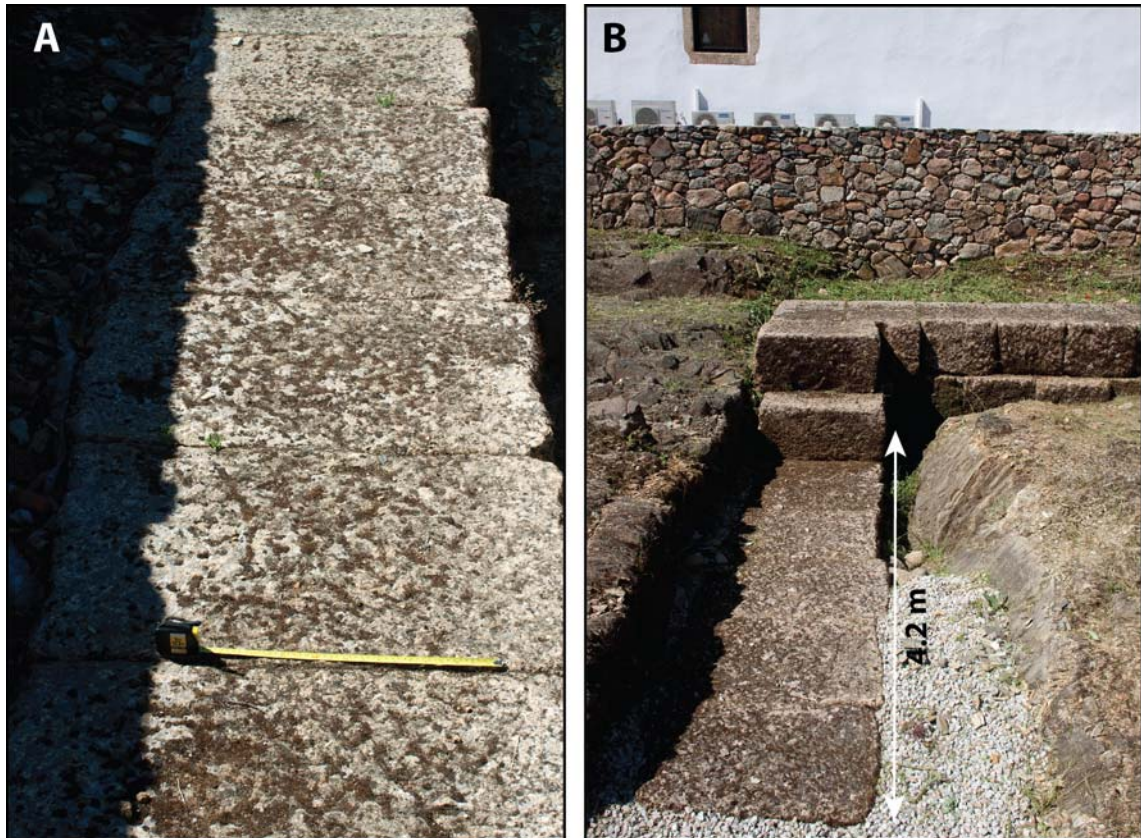
Figure 4.44 (A) Well-cut and smoothed granite ashlars used for the construction of the mausoleum (scale: 50 cm); (B) Free-standing foundation built into a U-shaped trench dug into the shale bedrock.
