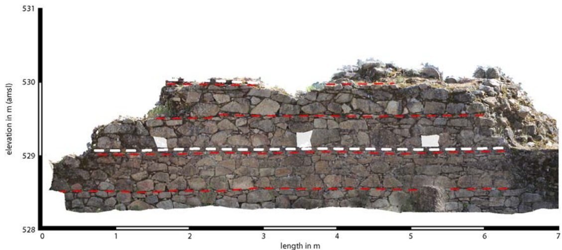
Figure 4.30 Orthorectified image of the eastern courtyard wall of the gate building. Levelling courses are indicated with a red dashed line, brick courses are indicated with a white dashed line.
