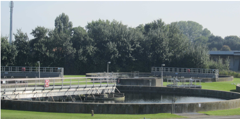
Figure 2.2: Circular secondary settling tank with central feed system and peripheral effluent overflow weir (WWTP of Roeselare, Belgium).
