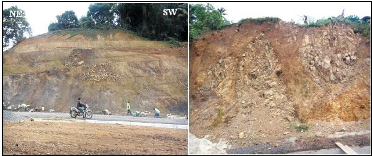
Fig. 2. 18. Profile of Bonjo slide exposed by road construction in 2009. Pale yellowish soil occurs on purplish saprolite. Note the presence of fractures, weathering heterogeneity and thickness of soil column.
