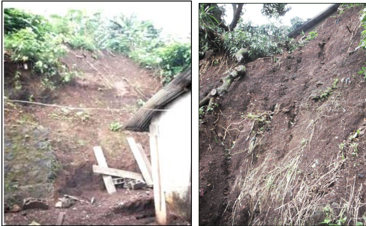
Fig. 2. 20. June 29 th , 2009 slide at Unity quarters, looking west. Note the presence of an uncompleted retaining wall west of the scar and steep slope created by material excavation for construction.
