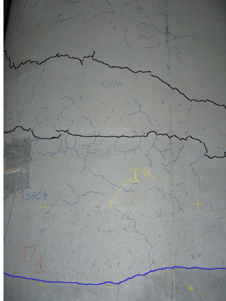
Figure 8.25: A network of cracks appearing in the HC, black lines are the main tangential cracks, blue line is the casting joint (Chapter 9)
