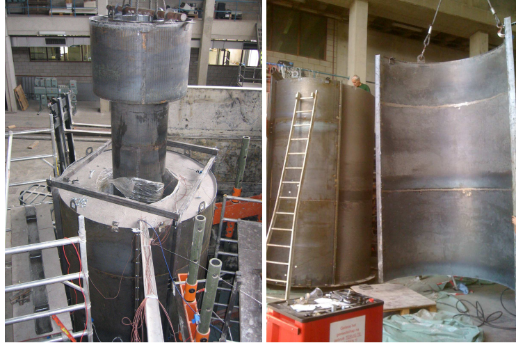
Figure 9.6: Uplift of the internal spill in between of the steel framework for the positioning of the LVDT's (left) and removal of the stainless steel formwork (right)
