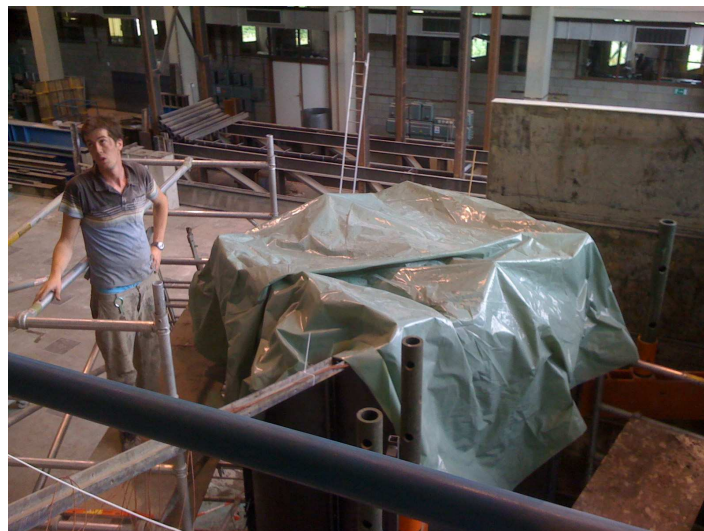
Figure 9.10: The first 68 hours after casting, a plastic sheet covers the Half-Scale Container
