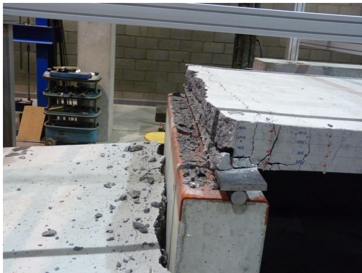
Fig. 23 Failure of the specimen due to complete rupture of the longitudinal reinforcement at the right inner support
