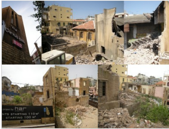
[Demolition of buildings on AYA-site. Images by author, taken in April 2010 and April 2011.]
