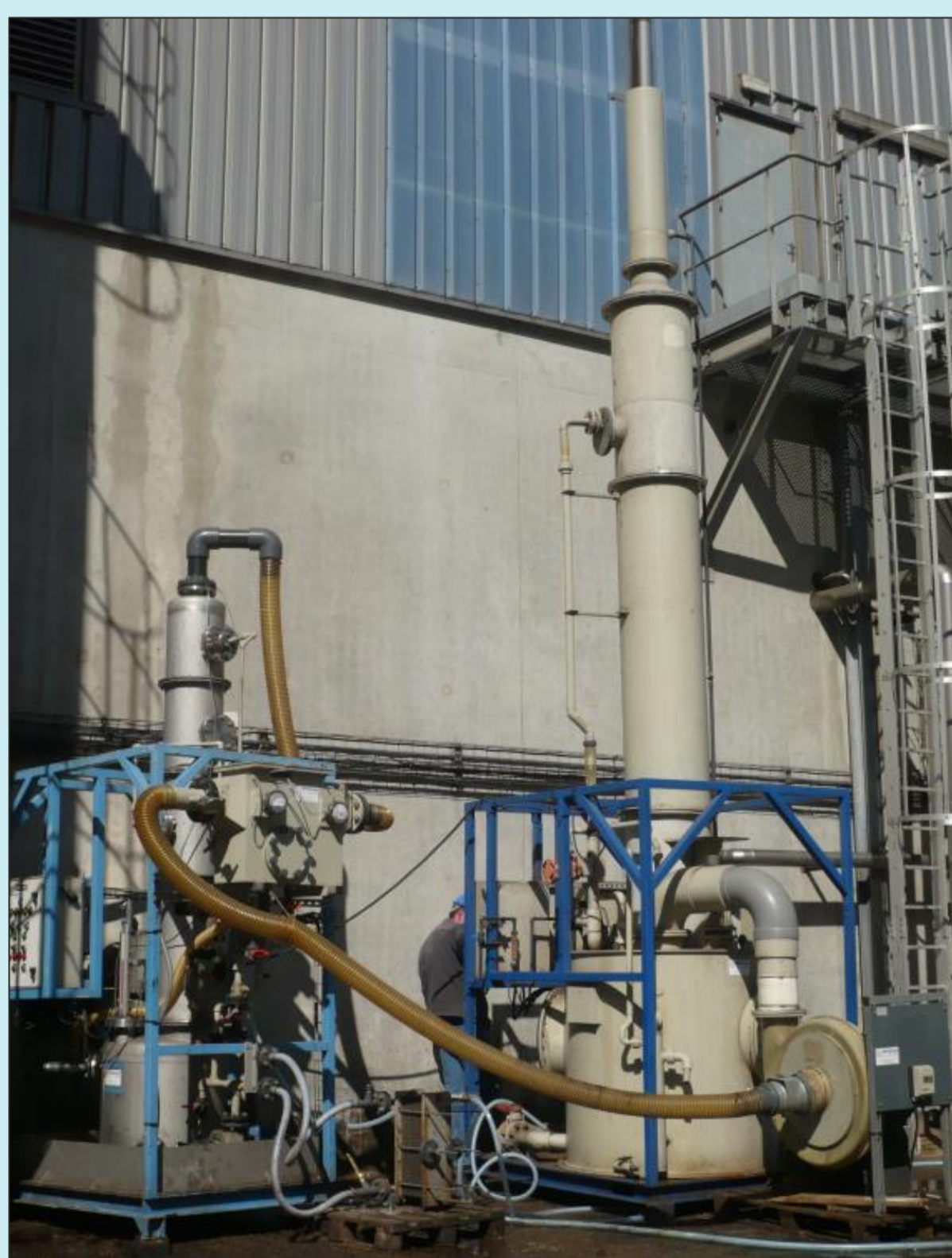
Figure 2. Ammonia stripping and scrubbing pilot at Waterleau, Ieper
