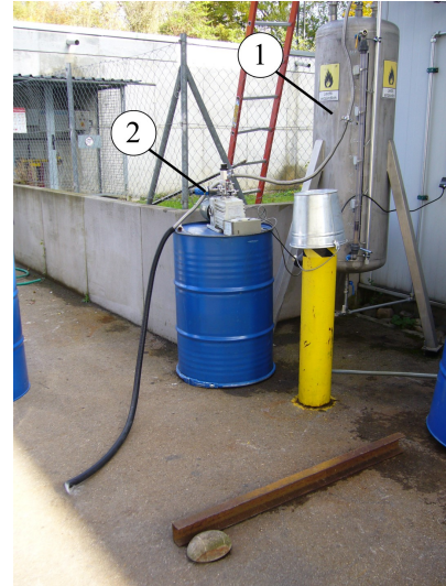
Figure 9: New vacuum pump fluid reservoir and membrane pump
