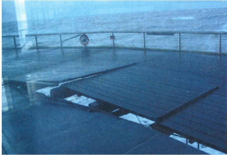
Figure 1.3 Wave uplift damage to outer walkway, 9 November 2007 (after Alderson & Allsop, 2008)
