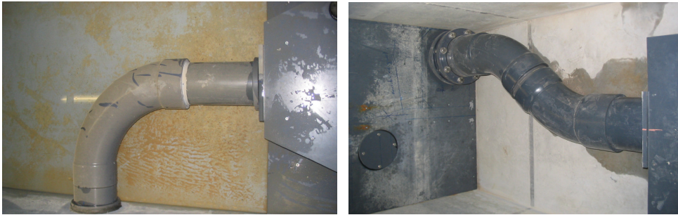
Figure II.4: Connection of the pipes with the in- (right) and outlet (left) structure
