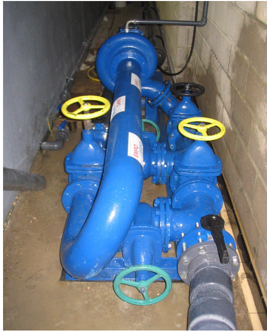
Figure II.3: Picture of the pump set-up
