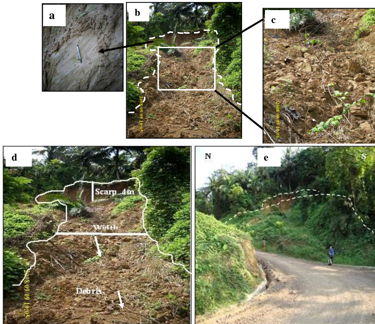
Fig. 2. 17. Field view of 2008 reactivation of the Bonjo slide; a) slicken slide at the head wall; c) detailed view slide debris; d) view of the 2008 reactivation of the 2005 Bonjo slide a week after slide reactivation. e) View of the July–August 2008 slide (photograph taken in November 2008). Note the backward migration of the head scarp and the degree of re-vegetation of slide debris three months after reactivation.
