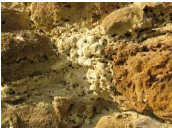
Figure 3: Detail of ferruginous sandstone masonry severely damaged by the perforations of mason bees.
