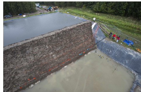
Figure 6. Total view at the end of the IJkdijk test with a completely filled upstream basin and minor sand deposits as a result of piping activity at the downstream side.
