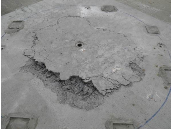
Fig. 7 Punching cone after fire test of slab S1 (top view)
