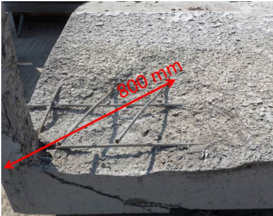
Fig. 11 Spalling damage of slab S0
