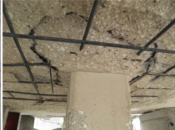
Fig. 8 Punching cone after fire test of slab S1 (bottom view)
