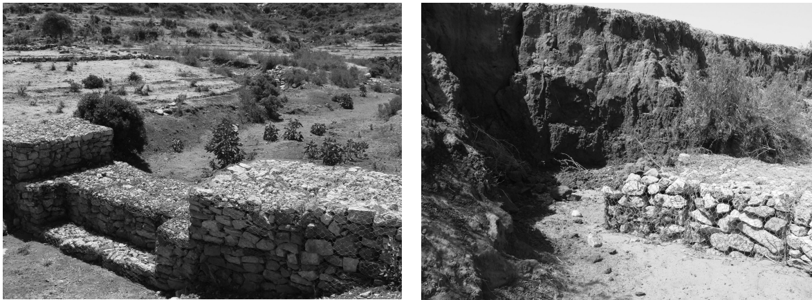
Figure 2: Gabions used to control gully erosion. Left: New gabion collecting a huge sediment deposit which could easily be used for vegetation planting. Right: Gabion bypassed by the flood. This could have been prevented by using appropriate complementary vegetative measures. (Photos © Reubens B.)
