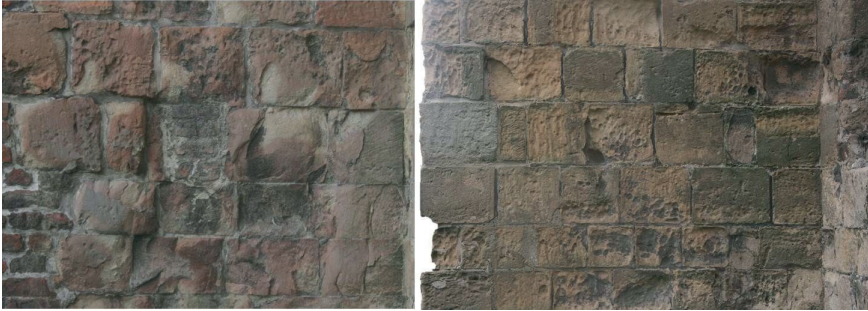
Figure 9.8: Macroscopic view (field of view approximately 1.5 \times 1.5 \text{ m}^2 ) of lower ashlar masonry of buff-coloured limestone with fissures and cracks, spalling, sanding, alveolization, soiling and red discolouration with large scaling.
