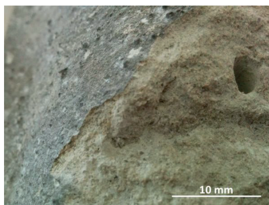
Figure 6.2: Cross-section photograph of Lede stone with gypsum crust from the Sint-Salvator church in Wieze.
