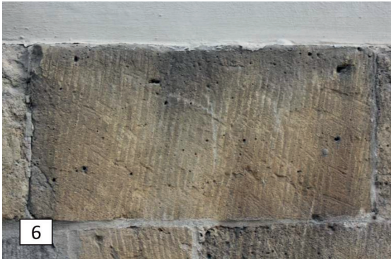
Figure 4.4: Photos 4–6 related to damage of white limestone.
