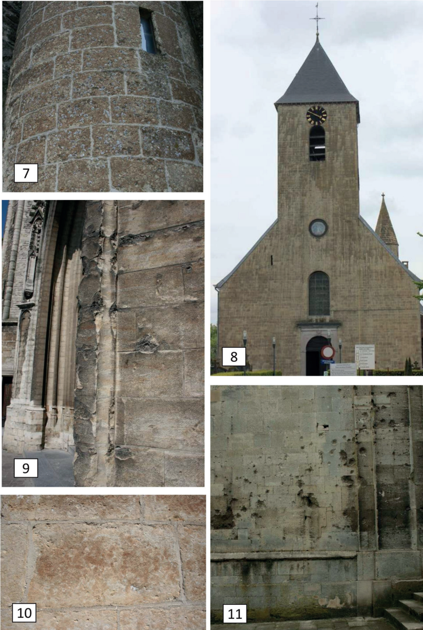
Figure 4.5: Photos 7–11 related to damage of white limestone.
