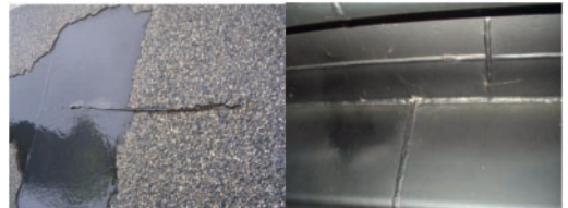
Figure 5. Longitudinal crack through the deck plate at a stiffener-to-deck plate connection (left), multiple welds intersecting at the crack location (right).
