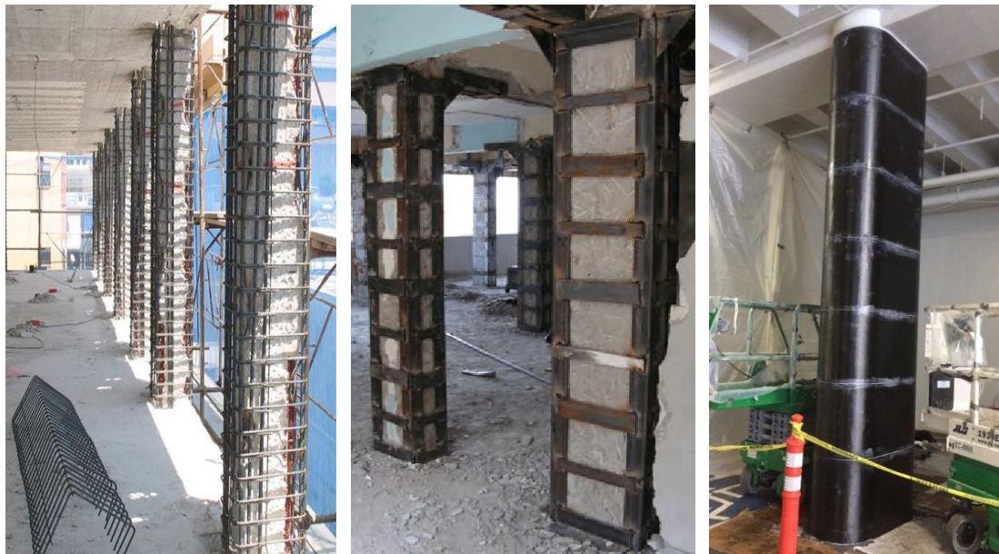
Figure 2.16: Different RC column strengthening/repairing techniques; RC jacketing, steel plate jacketing and FRP jacketing, respectively.
