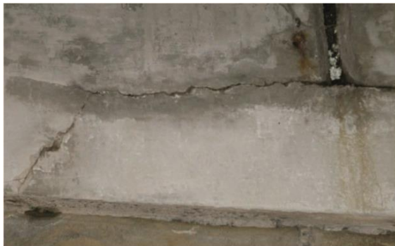
Figure 4: Superstructure cracking (BAST, 2015)
