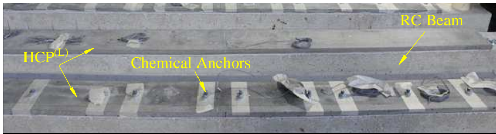
Figure 6.8: Images of some of the beams after fixing the strengthening plates (note that beams are positioned upside-down)
