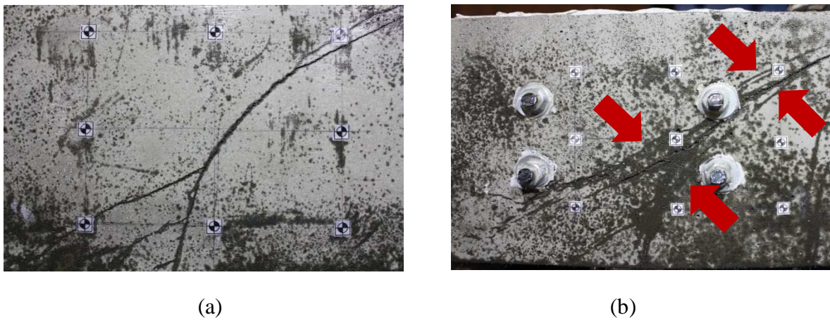
Figure 4.39: Close-up views of the major diagonal crack caused the failure of the beam (a) BS_A, and (b) BS_AB (arrows are indicating the band of cracks)
