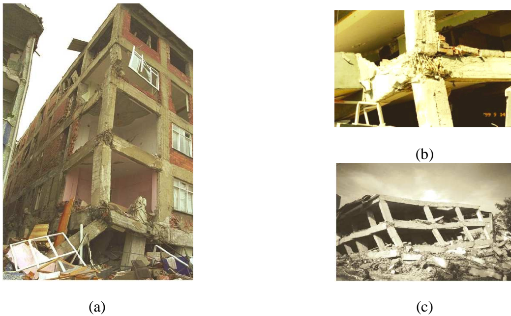
Figure 2.28: Failure of beam-column joints observed in the 1999 İzmit, Turkey earthquake (photo credits: (a) Courtesy of National Information Service for Earthquake Engineering, University of California, Berkeley, (b) Prof. Güney Özcebe, personal communication (1999), (c) Said and Nehdi [81])
