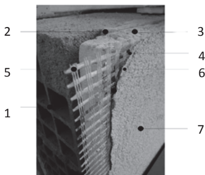
Figure 4. Components of a ETICS system: 1) base wall 2) Adhesive Layer 3) Insulation Board 4) Regularization layer 5) Rendering 6) Regularization Primer layer 7) External Coating (Plaster) (Perdigão, 2013).
