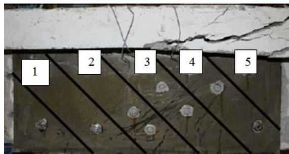
Figure 3-34: Final crack pattern of the R-SP-5L45-III beam
