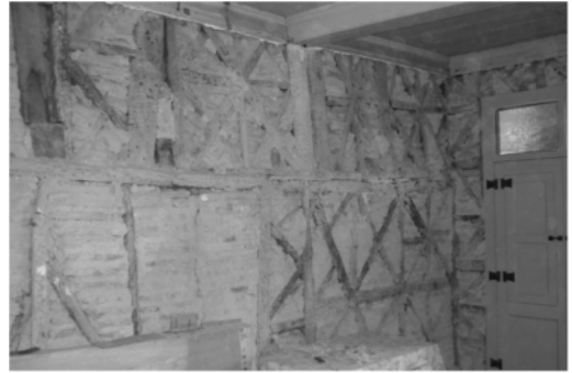
Figure 4. Timber frame walls in a traditional house in Guimarães (credits: E. Poletti).
