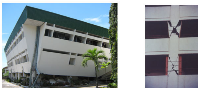
Fig. 1 - Negative effects of infill panel in structure; soft story mechanism [12] (left), short column mechanism [13] (right)
