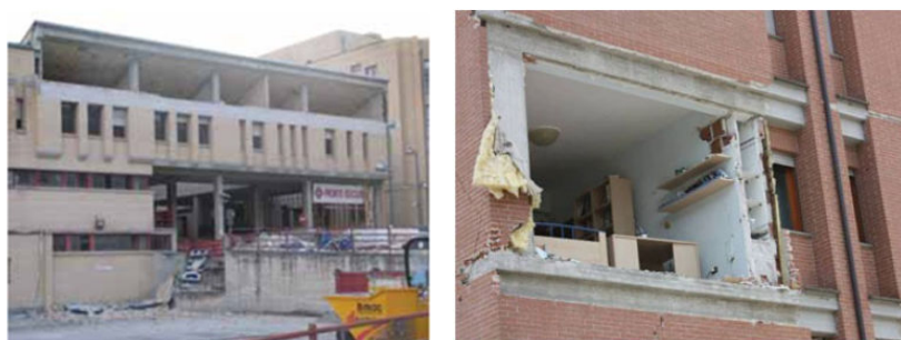
Fig. 2 - Damage in non-structural elements [2]
