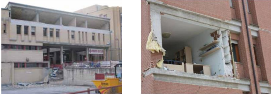
Figure 2 Damage in non-structural elements (Braga, Manfredi et al. 2011)
