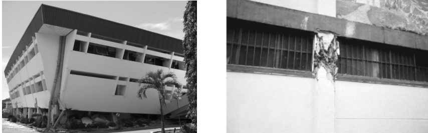
Figure 1 Negative effects of infill within structure; soft storey mechanism, (Kusumastuti 2010)(left), short column mechanism (Guevara and García)(right)
