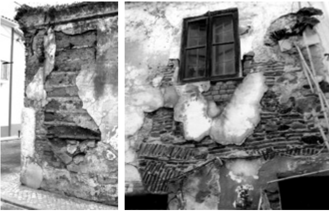
Figure 2. a) Horizontal rammed-earth reinforced with fired brick, Benavente . b) Relieving arches in Alcácer do Sal , Portugal (credits: CI-ESG).
