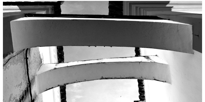
Figure 6. Historical centre of Évora , placing of counter-arcs between the different blocks (credits: CI-ESG).
