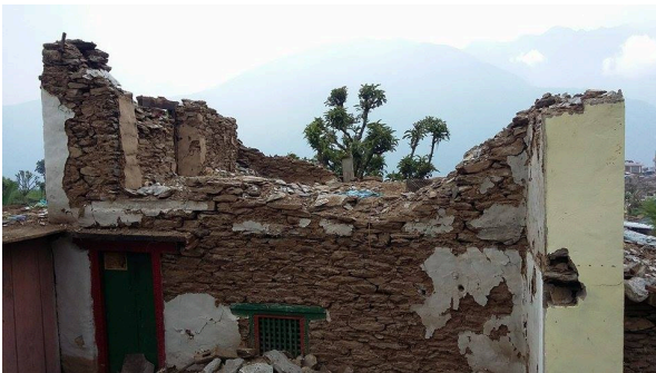
Figure 11 – Collapsed house with a heavy roof during the Gorkha earthquake, 2015 ©DipendraGautam 2015
