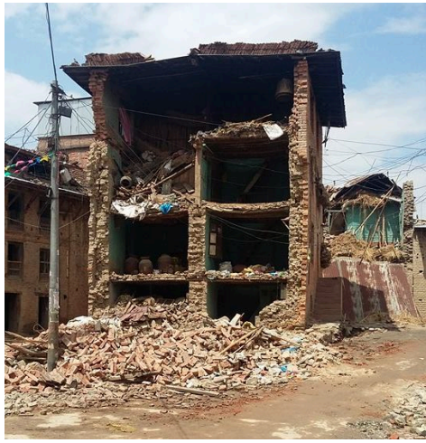
Figure 10 – Out-of-plane façade failure during the Gorkha earthquake, 2015 ©DipendraGautam 2015
