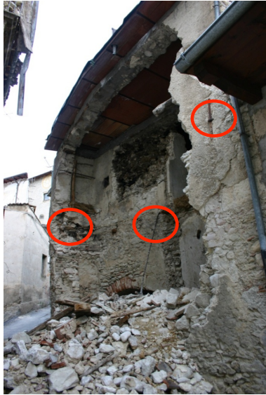
Figure 6 – Collapsed façade of a building with ties, during L'Aquila earthquake
