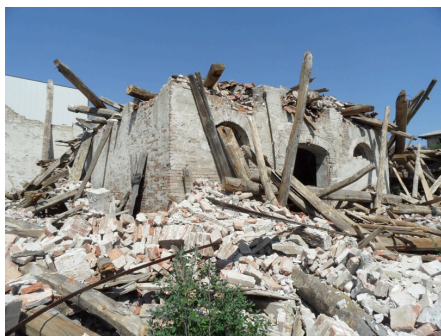
Figure 7 – Masonry buildings collapsed during the Emilia-Romagna earthquake
