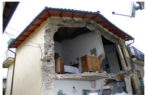
Figure 5 – Out-of-plane collapse of a façade masonry wall
