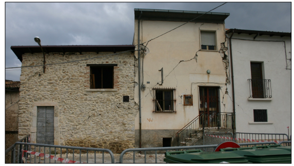
Figure 12 – Damage associated to the interaction between adjacent buildings - L'Áquila earthquake
