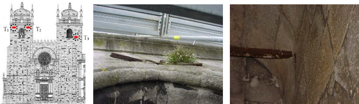
Figure 5: Ancient tower ties, with deformed anchorage ( T_1 ) and broken tie ( T_3 ).
