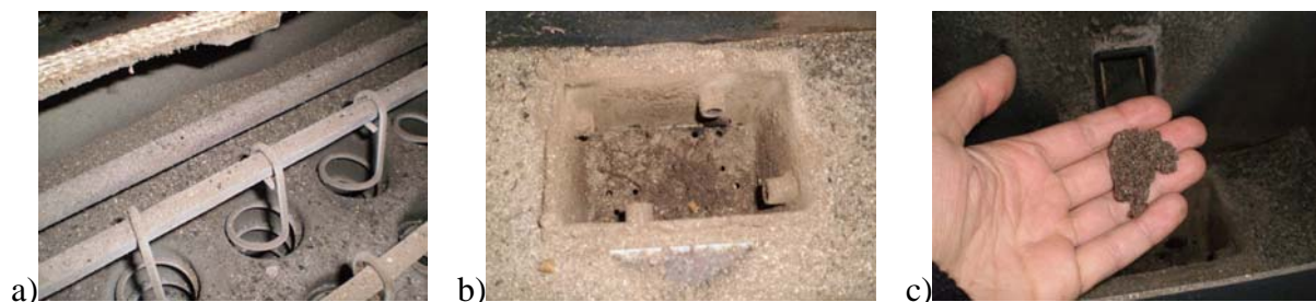
Figure 3. Ash problems in the boiler by the FRWP: a) fouling in the heat exchanger; b) slagging and obstruction of the air inlets of the grate; and c) slagging of the ash fusion.
