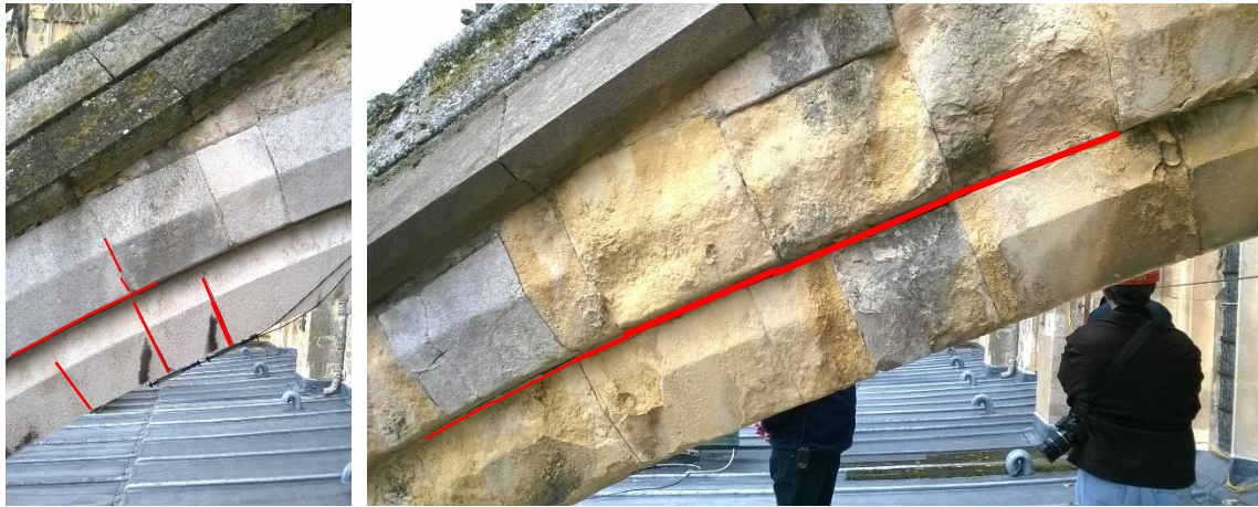
Figure 4-11. Crack patterns of joint failure from west view of flying buttress 2 (Left) and 3 (Right) of the south aisle of Canterbury Cathedral.
