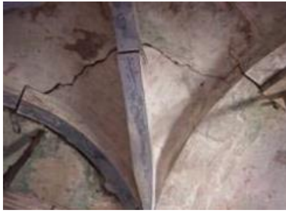
Figure 4-6. Corner detachment of a vault, provoked by differential settlements and rotations at base, in the Monastery of Salzedas, Portugal (Lourenço et al. 2008).
