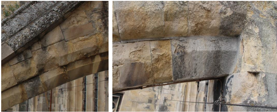
Figure 4-12. Crust formation and flaking in large areas of Caen stone masonry from west views in the flying buttress 3 of the south aisle of Canterbury Cathedral.
