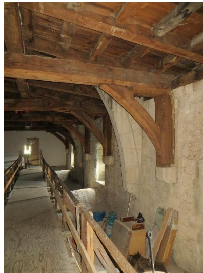
Figure 3-13. View of the roof void in the south aisle looking west (Photographic survey).
