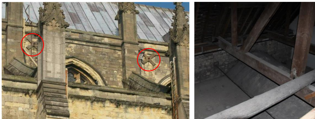
Figure 3-14. (Left) External view of the nave clerestory walls of Canterbury Cathedral, depicting the two anchor cross shaped plates on the right side of each transverse section (Morton Partnership Ltd). (Right) Inside view of the roof void in the nave of Canterbury Cathedral, depicting the iron tie in the clerestory walls above the vaults (Photographic survey).
