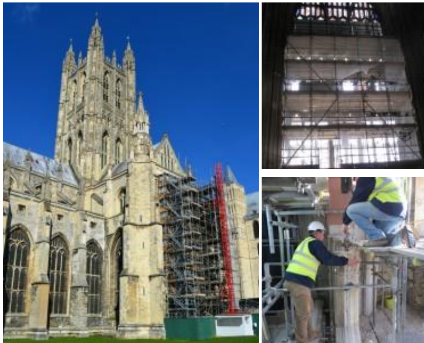
Figure 2-39. (Left) The Great South Window of the South West Transept behind scaffolding. (Right above) Inside view of the Great South Window tracery of the South West Transept. The glass panels have been removed and stone parts are been taken off piece by piece. (Right below) Process of removal of damaged stone masonry in the Great South Window tracery of the South West Transept which will later be replaced by replicas. View of the tracery at top level. ("The Great South Window" 2014).
