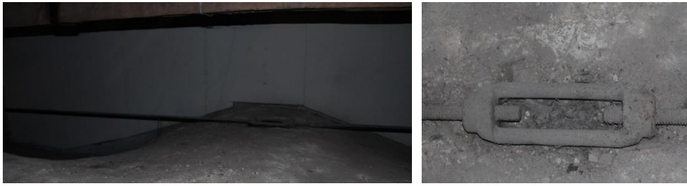
Figure 3-15. (Left) View of the iron tie at mid span (Right) Coupling system at the mid span of the iron tie (Photographic survey).
