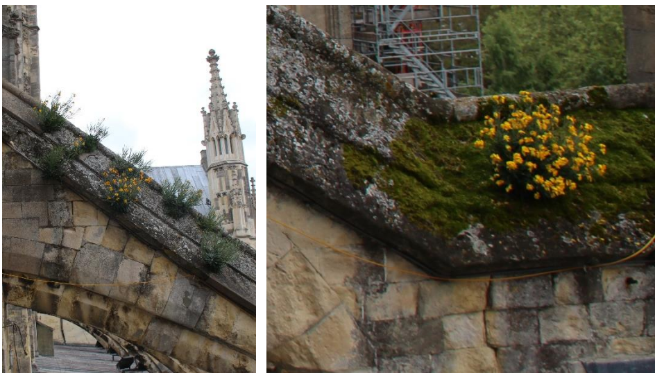
Figure 4-13. Biological growth in form of algae, mosses and higher plants in the upper surface of flying buttress 3 (east view) in the south aisle of Canterbury Cathedral.
