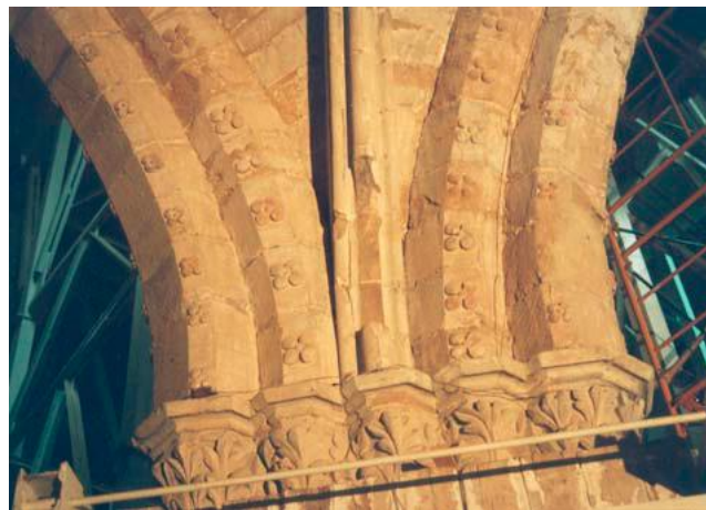
Figure 2-24. Pier of Tarazona Cathedral. Under excessive compressive stresses stone crushing and detachment occurred (Roca et al. 2005)
