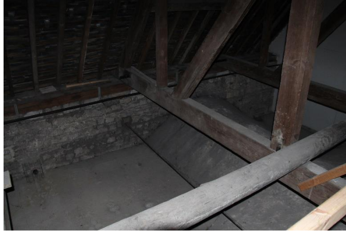
Figure 2-38. View of the interior nave roof void, depicting the concrete infill layer and the drilled hole for drainage.
