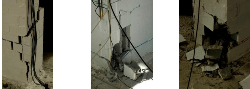
Figure 3.13 – Damage in corners during the test of 250%
