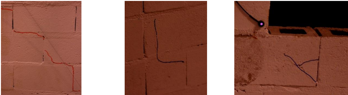
Figure 3.7 – Damage in the middle of the walls affecting unit blocks
