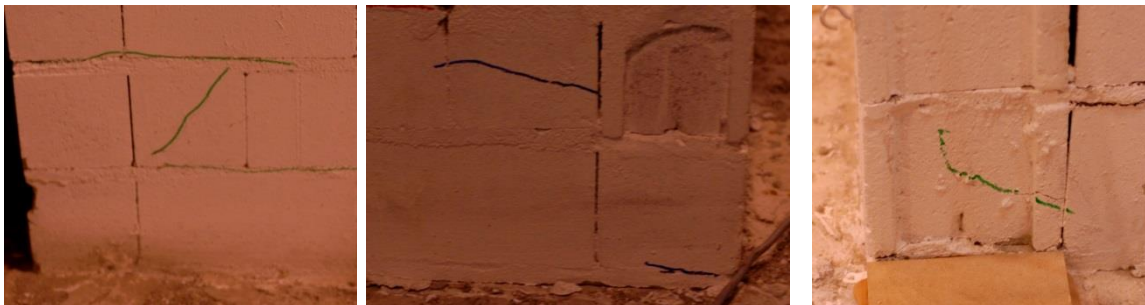
Figure 3.8 – Damage at the bottom of the walls, mainly at corners affecting unit blocks
