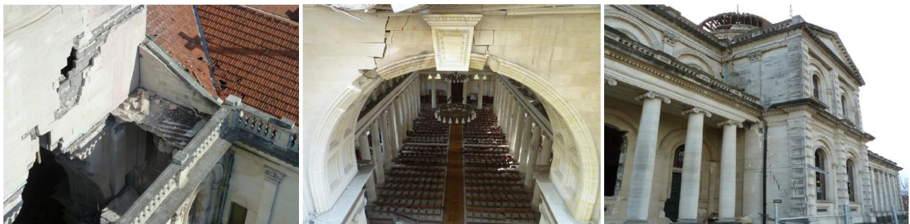
Figure 5. Collapse of a North of the adjacent RC flat roof and interior arch (left); Damage along the West arch (middle); Developing of a diagonal block failure in the South transept façade (right).
