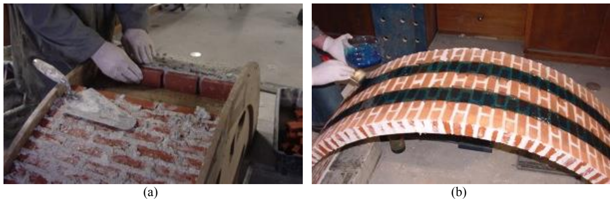
Figure 1: Masonry arches preparation: (a) bricks assemblage near the key stone during construction and (b) finished specimen after 1 week of curing, during application of GFRP strips.
