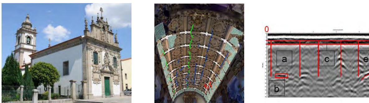
Figure 6 – Details of the St. Vincent Church in Braga - elevation (left); damage and deterioration in the main vault (center); GPR inspection (right).
