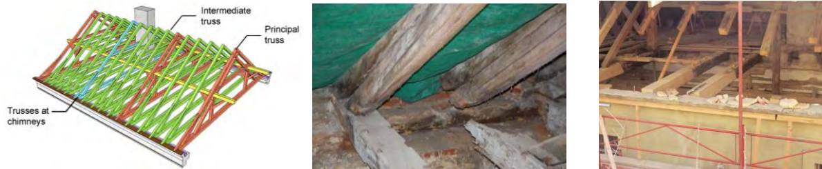
Figure 5 – Schematic of existing roof system (left); rotted ends of trusses (center); timber repairs during restoration (right)
